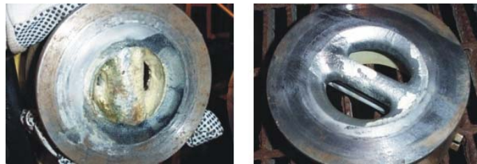
Heavy Scale Build Up After 3 Months Without MFC's Installed
