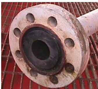
Tubes are clean after 15 months with MFCs installed.
