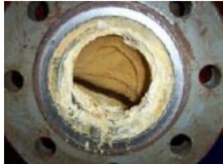
Oil control valve after three months without magnetic fluid conditioners installed.
