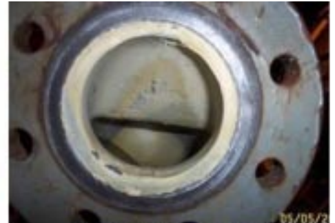
Oil control valve after eight months with magnetic fluid conditioners installed.
