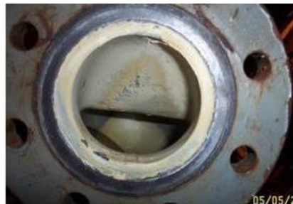
Oil control valve after eight months with magnetic fluid conditioners installed
