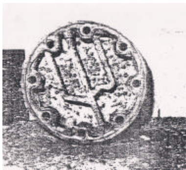
FIGURE 6, TEST AIR CONDITIONING CONDENSER JULY 1990 SHOWING END PLATE CONDITION NOTE: NO CLEANING DURING TEST PERIOD (23 MONTHS)
