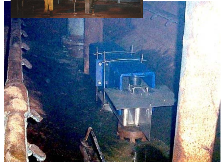
Scale-X ® magnetic fluid conditioner installed in Petronas Carigali separation vessel
